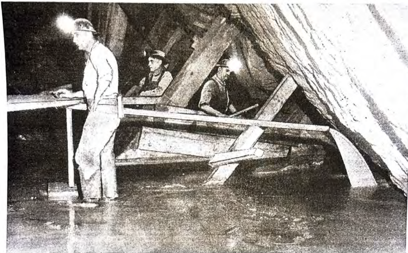
FRESH SAND-SLIME FILL is solid enough to permit the operator Raymond Coulter to stand on it. The fill is discharging from the pipeline at the right. In the background, two miners are just completing a cribbed raise that comes up through the fill.
