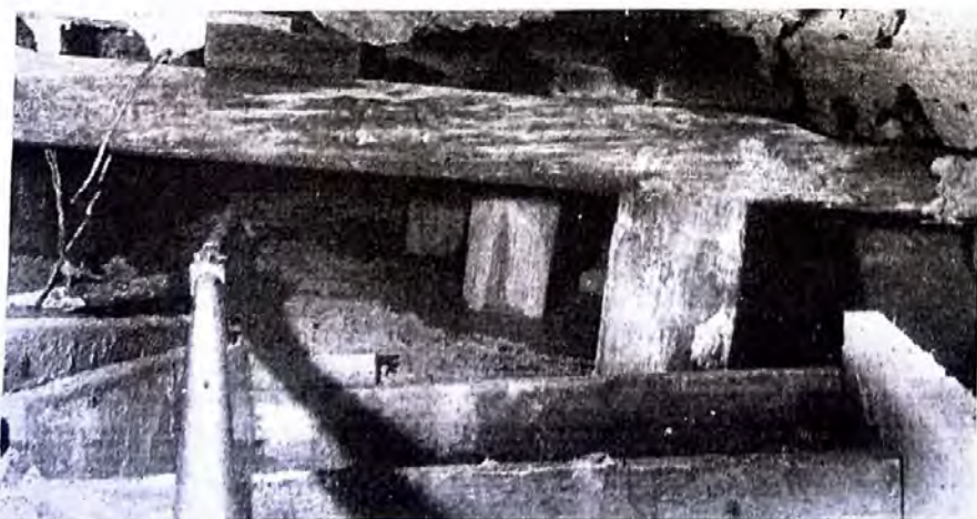
TAILINGS FILL close to back of old timbered stope. In foreground is timbered raise. Stretching away from camera is pipeline that conveys the sand-slime fill.
