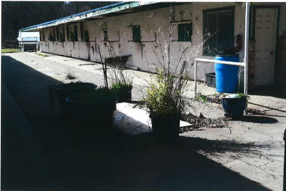
4G. The existing septic tank is beneath the plywood next to the planter containers shown in this photograph.
