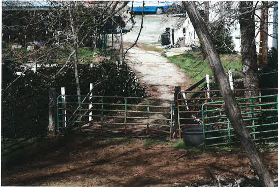
4A. View to the north showing the existing road and bridge over French Ravine Creek.
