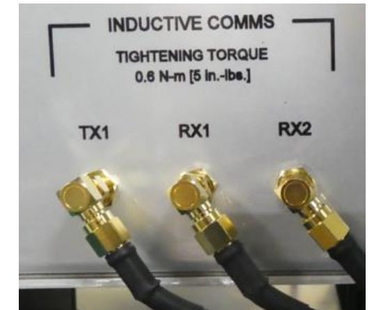
Figure 4: Inverter RF Terminations 4X
