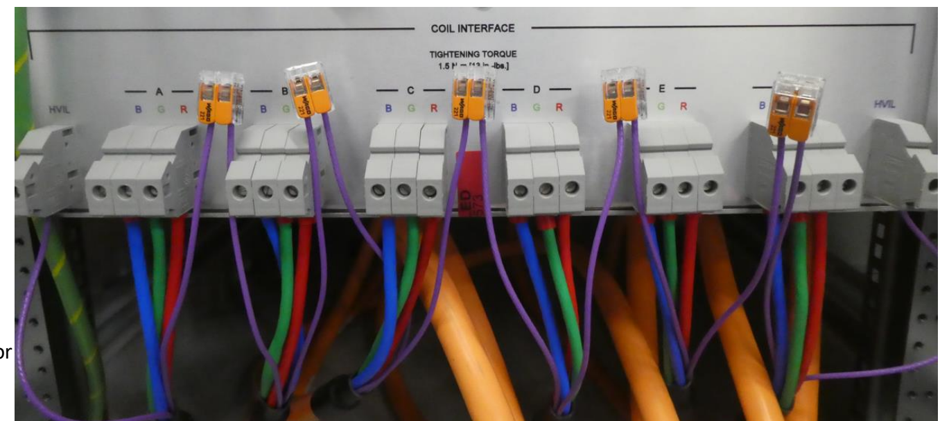
Figure 12: Bottom Inverter Litz Cable Connections
