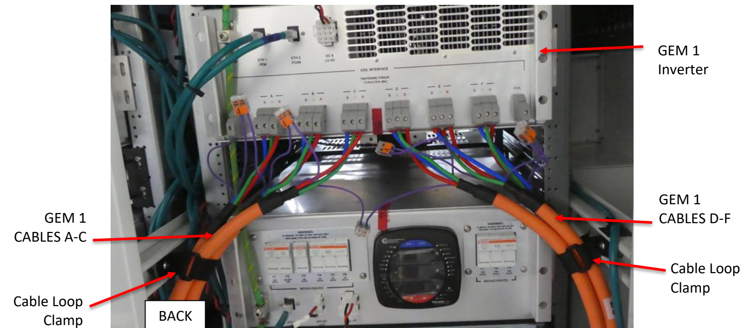
Figure 14: Top Inverter Litz Cable Connections
