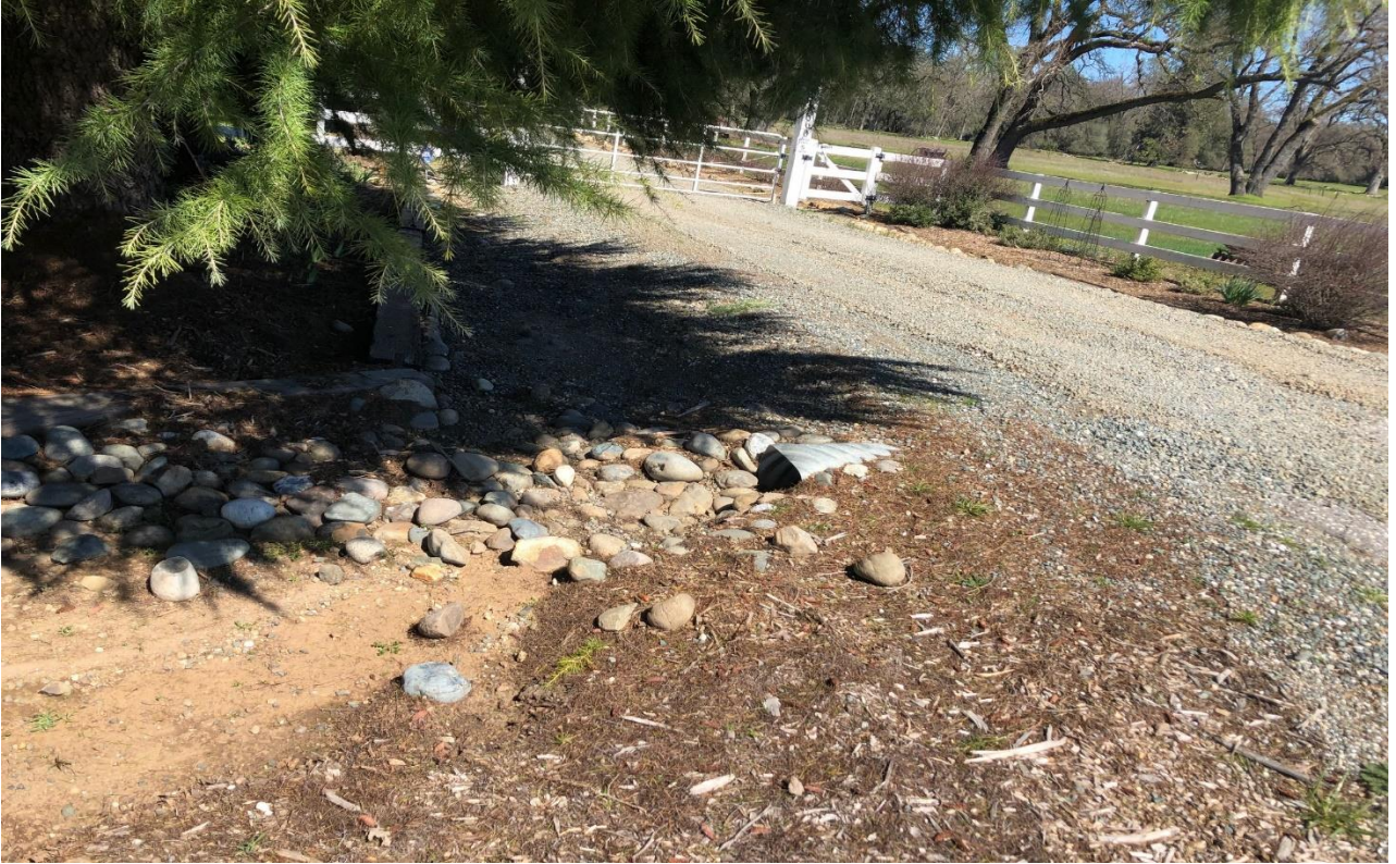
Photo 7: Rock lined driveway drainage with culvert. Drainage feature does not contain defined bed and bank, ordinary high water mark, or a direct connection to any other stream up/downstream.
