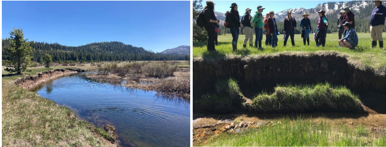
Figure 2: Spring runoff on the South Yuba River is constrained within the channel (left). Lyton Creek's banks are actively sloughing and eroding (right).
