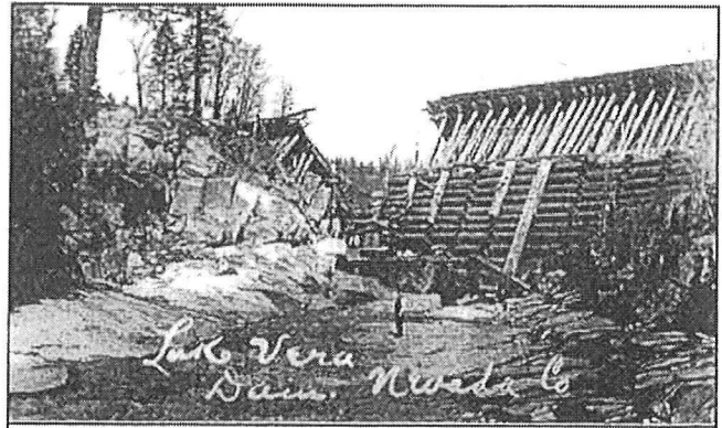
The Lake Vera Dam was originally 54 feet high and it failed in early 1905, as this photo shows.
