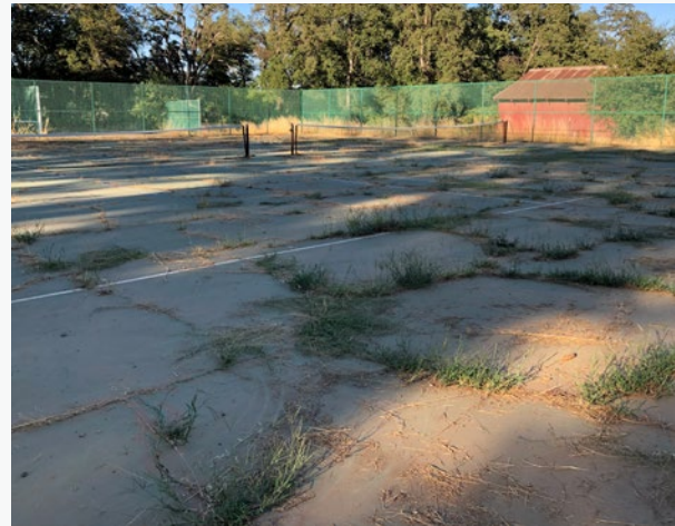
Tennis/pickleball courts are weeded by volunteers but are in need of significant repair.
