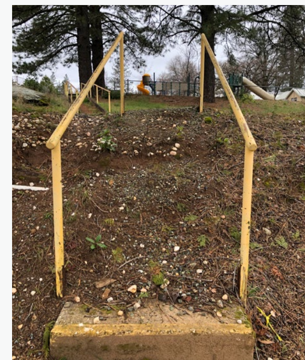
Stairs and pathway connections between Oak Tree Community Park and the Family Resource Center pose a safety hazard and are in need of renovation and repair.
