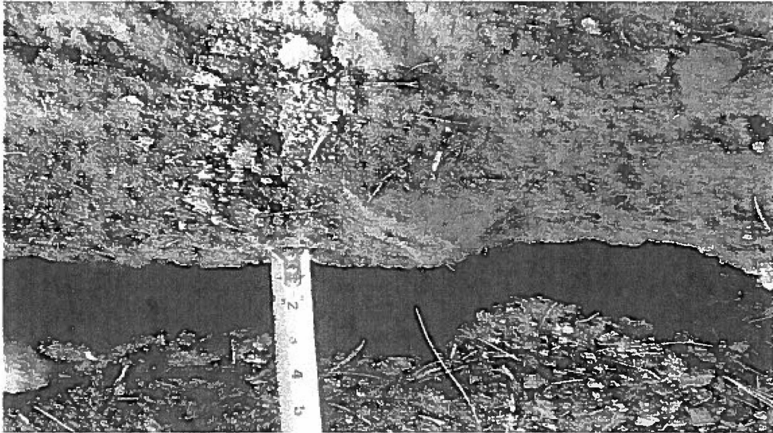
Photo 9 – Measurement of soil crack adjacent to Pasquale Road residence (APN 38-240-16).
