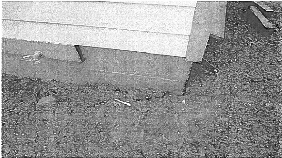
Photo 10 – Developing crack along foundation (APN 38-240-14).
